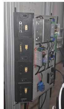
Fig. 3. ECS BOX power management system.
